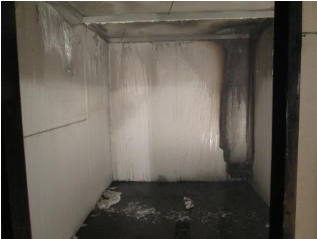
Photos Immediately After Test
