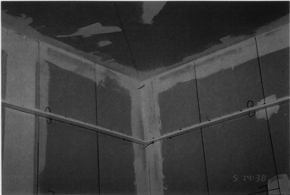
Figure B-1. View of Crib Corner at the Wall/Ceiling Intersection. Aluminum Angle is Mounted 12 in. Below Gypsum Ceiling Around Interior of Room.
