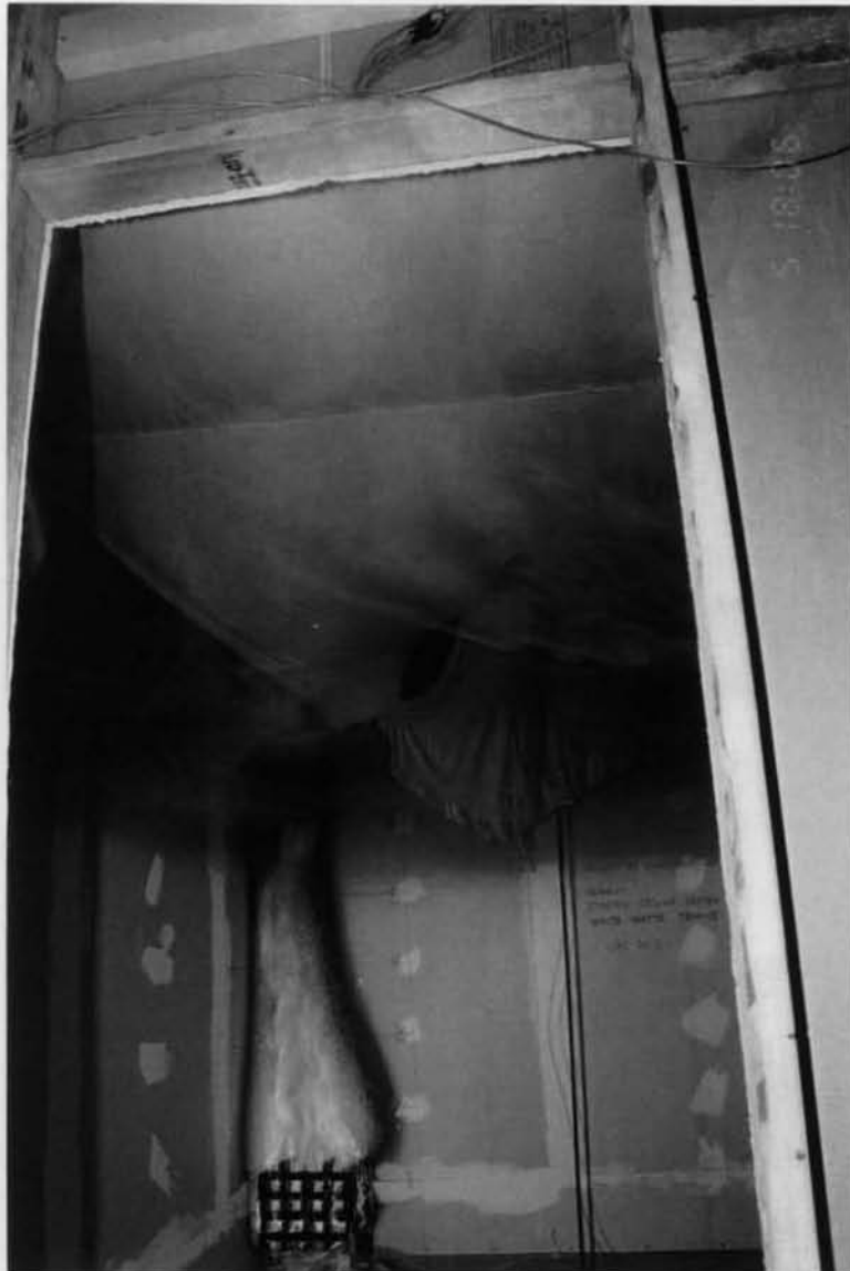
Figure B-9. Room Interior at Approximately 14 Min into 15-Min Fire Exposure. Reinforced PVC Membrane Is “Hanging Down” Approximately 2½ Ft Down from 8-Ft Ceiling (5½ Ft Above the Floor).
