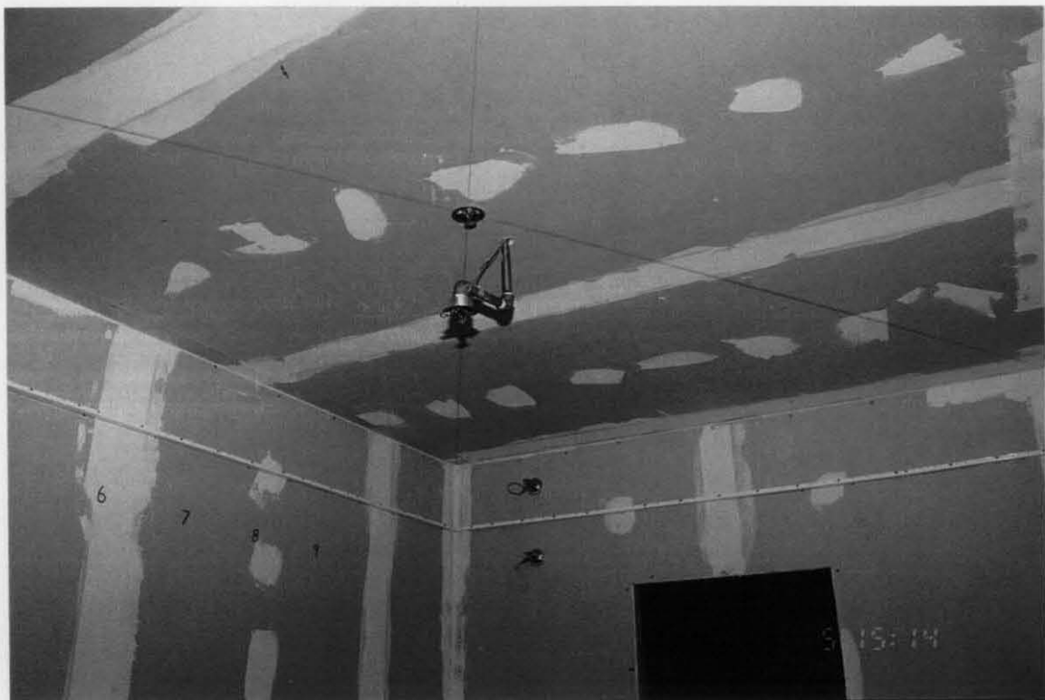
Figure B-2. Room Interior Ceiling with Sprinkler Heads Installed Before Installation of Reinforced PVC Membrane.
