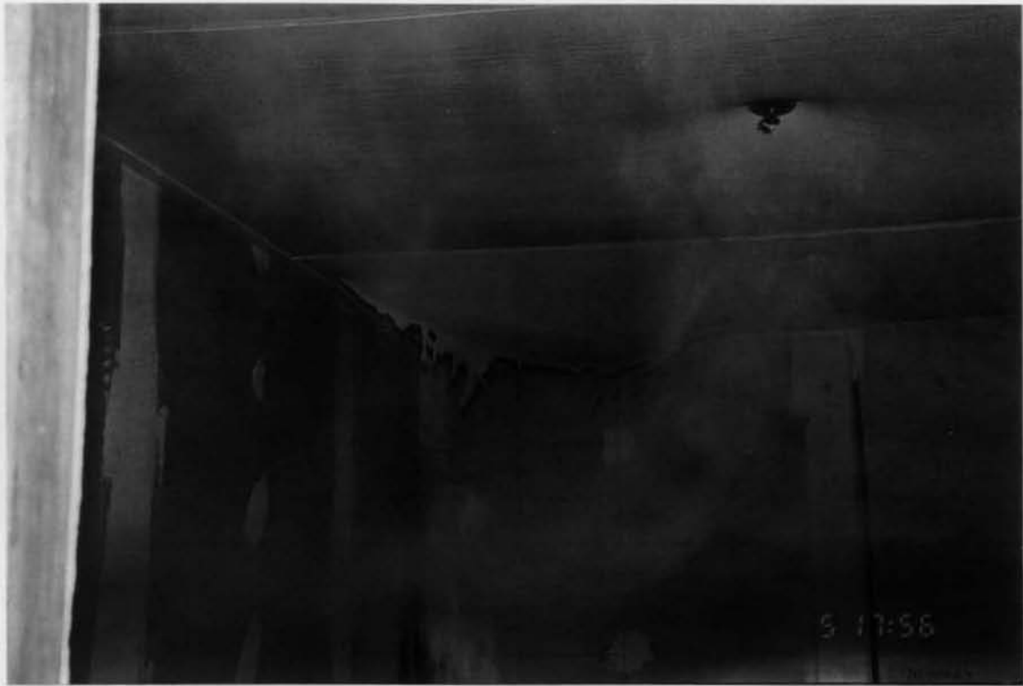
Figure B-6 View of Test Corner and Ceiling. Reinforced PVC Membrane Is Beginning to Sag at Crib Corner and Around Sprinkler Head.
