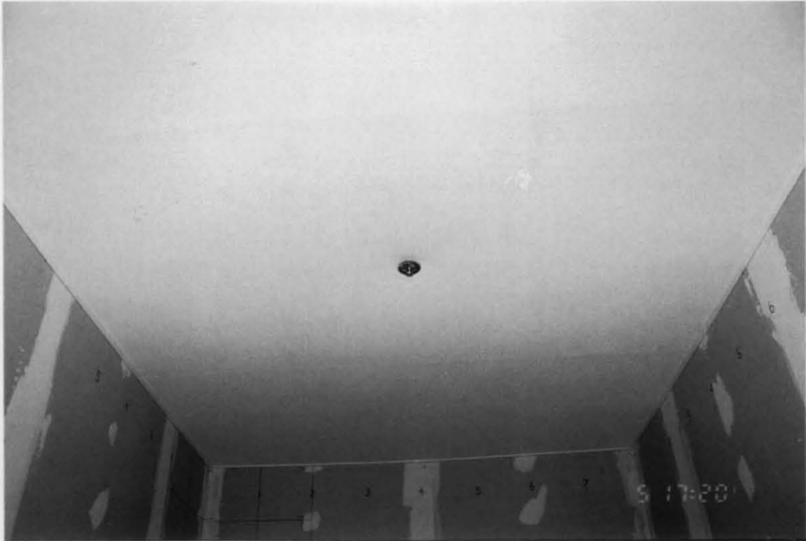
Figure B-3. View of Reinforced PVC Membrane with Flush Mount Sprinkler Head Installed at Center of Room.
