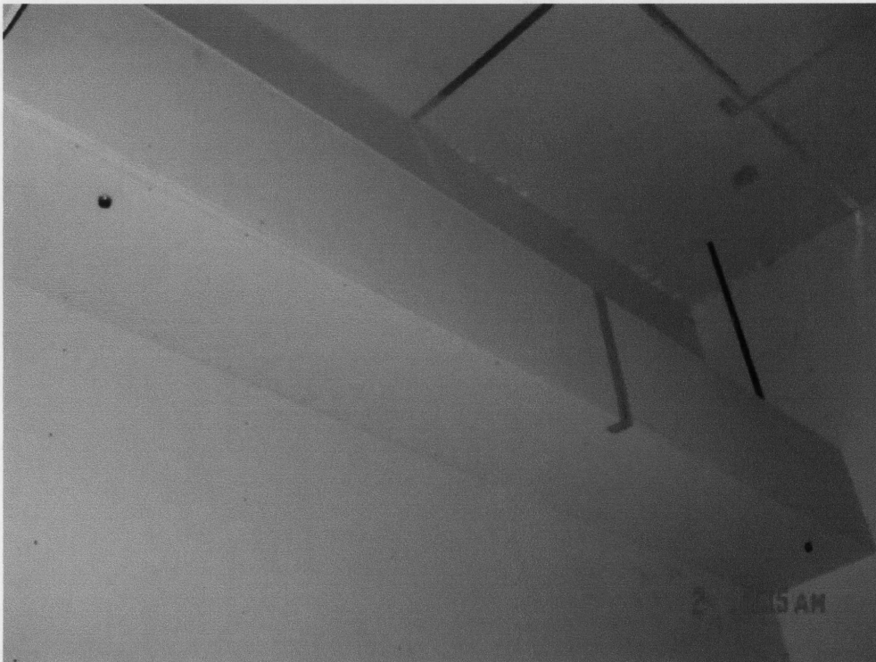
Photo 4: Soffit on Left Side of Room: Sprinkler #1 on the Left and #2 on the Right.
